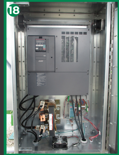
DC shield removed to show detail
