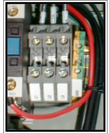
Electrical connection terminals.
